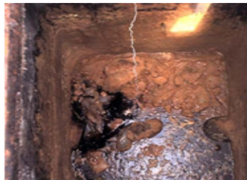
Pumping well with a build-up of solids
