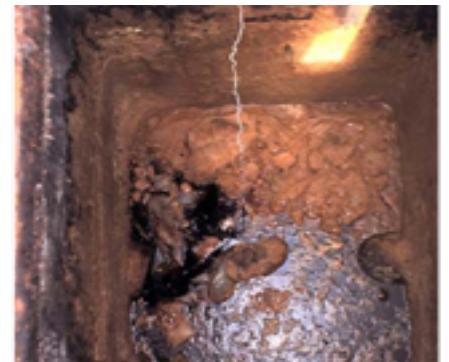
Pumping well with a build-up of solids
